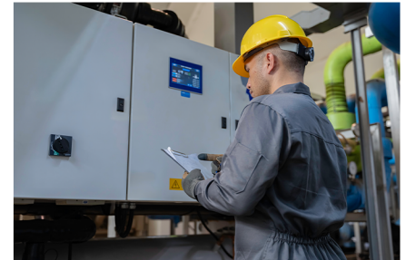
Control panel evaluation: wiring, labeling, and protection
