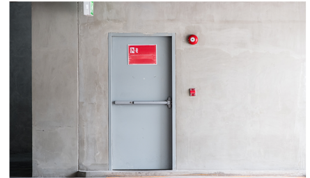
Fire Door Compliance Evaluation and Inspection
